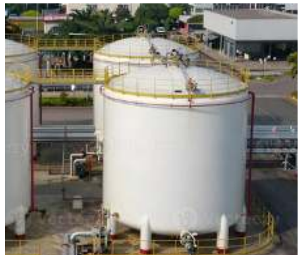
LPG Storage Tanks
